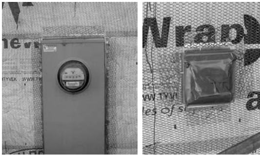
Illustration 3: Electric Meter and Fan Vent
